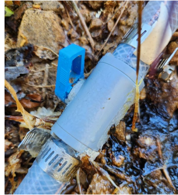
Gravity feed caustic control
