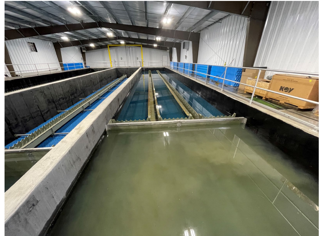
Rectangular clarifiers at Buffalo Coal (S-2003-88) which is like the design for LFLS clarifier.
