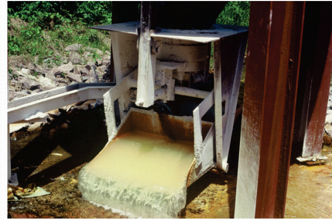
Tipping Bucket Lime Feeder
