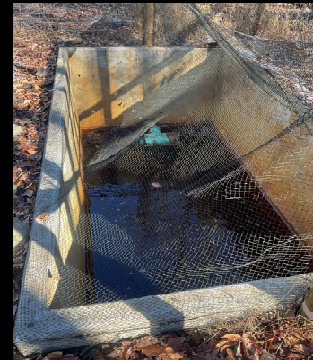
Grit Chamber to Settle Out Iron
