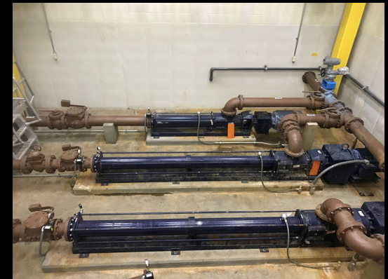
(5) Sludge Pumps to Mine or Geotubes
