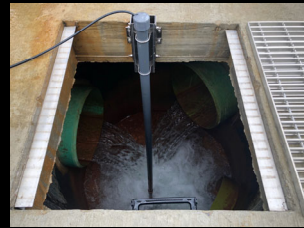
(3) Mix tank pH monitoring and polymer injection
