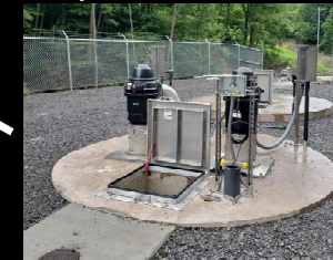
1200 GPM Lift Station to Plant
