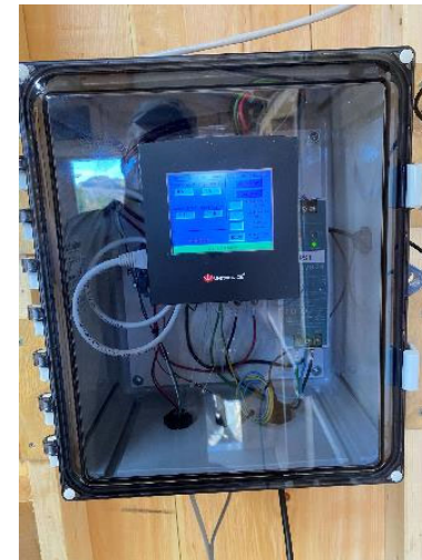
PLC Based pH- Controlled Pinch Valve System for NaOH Addition
