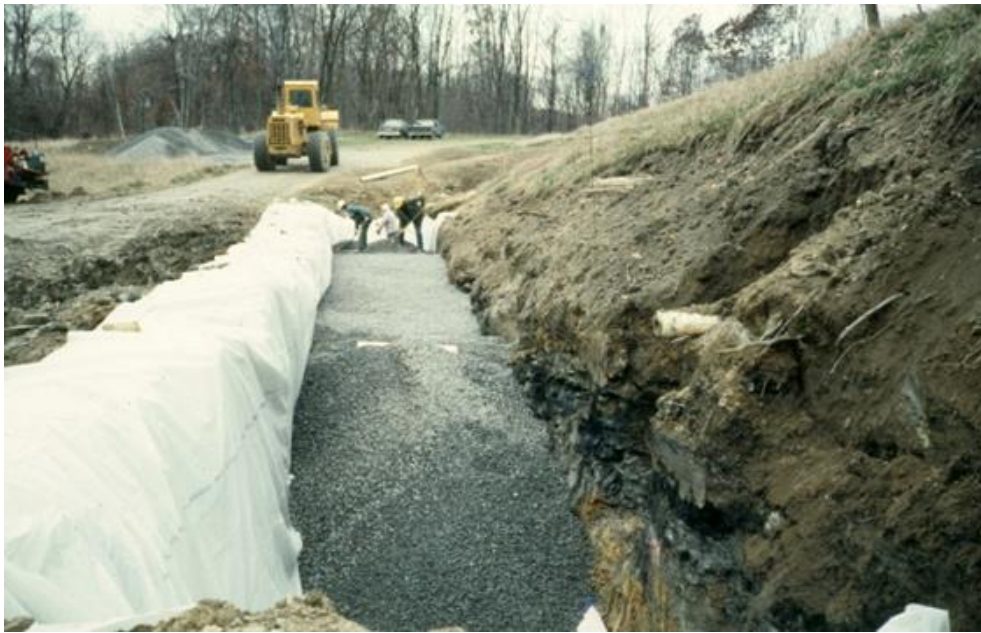
Figure 5. An anoxic limestone channel being constructed, soon to be covered with plastic sheeting and a soil cover.
