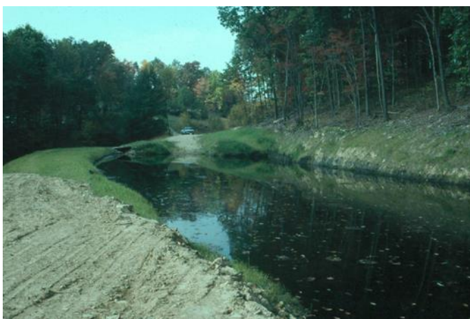
Figure 6. Construction of an early SAPS in 1995, which has subsequently also been referred to as RAPS, vertical flow ponds, and vertical flow systems. A. Initial placement of the limestone base layer with underdrain piping. B. Compost layer being placed on top of the limestone. C. The system filled with water.
