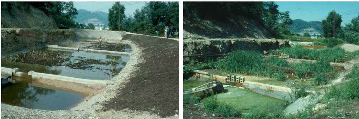
Figure 3A. A Typha-based wetland immediately after construction in West Virginia. B. the same site, two months later.
