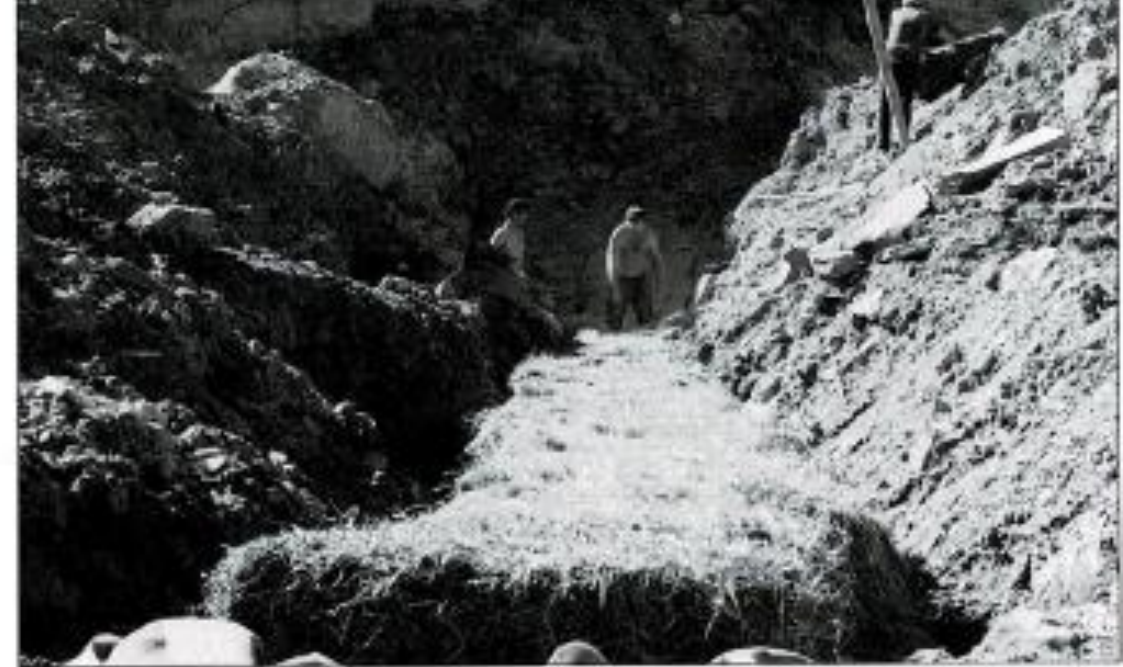
Figure 2. Hay bales were placed on top of the filter fabric lined trench filled with limestone.
