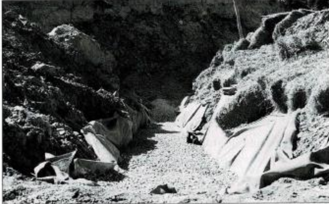
Figure 1. Excavation of the trench was followed by placing filter fabric in the trench, and then filling the trench with limestone.
