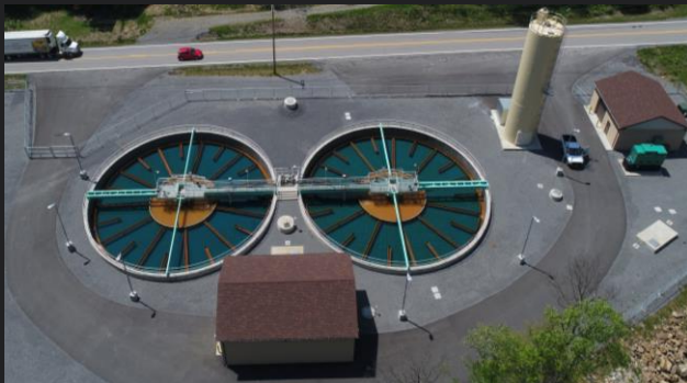
4,200 GPM AMD Treatment Plant
