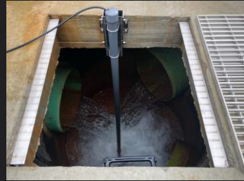
(3) Mix tank pH monitoring and polymer injection
