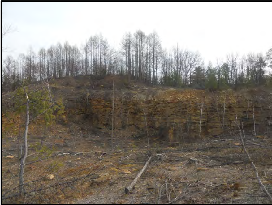
Figure 18 – Pre-Construction 2012 Typical Dangerous Highwall
