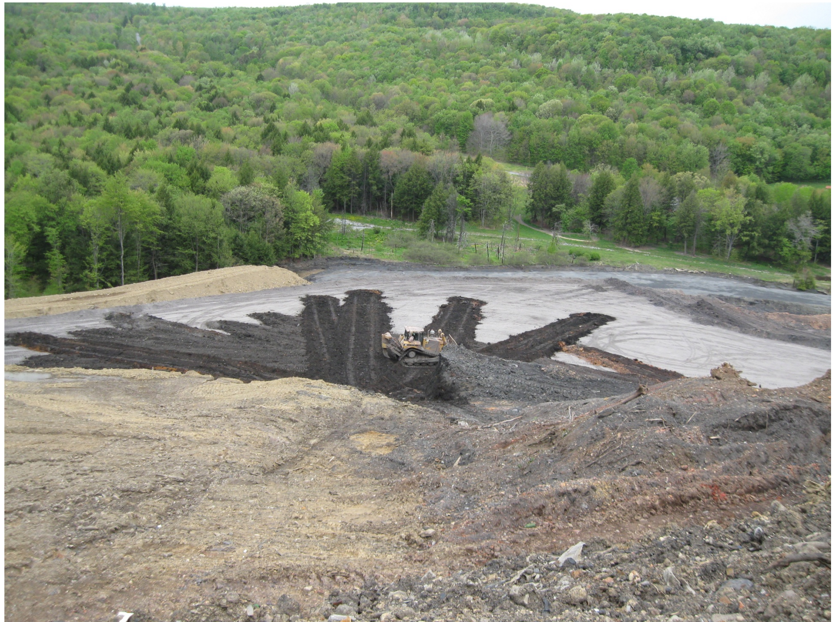
Reject refuse material being spread on top of a layer of ash Photo from Nanty Glo West on May 7, 2010
