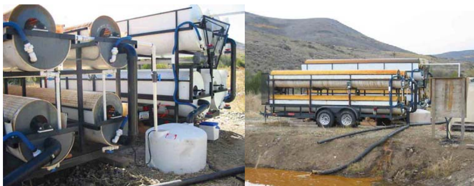
Figure1. The 600-gallon capacity and 1200-gallon capacity units at the Rio Tinto Mine Site
